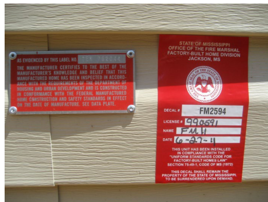
Figure 1. Inspection Decal Placed on the Exterior of the Home Near the HUD Label.
